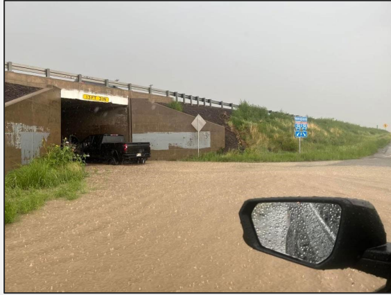
Photo 1 : Taken from west side of I-25a looking southbound. Significant flooding frequently occurs during storm events due to poor drainage.
