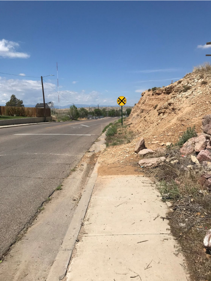
Sidewalk stops before RR crossing, forcing pedestrians to merge with vehicular traffic.
